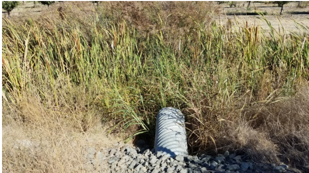
Photograph 3. Culvert emptying into the agricultural ditch from across Wilson Road (facing north) Taken on September 30, 2016.
